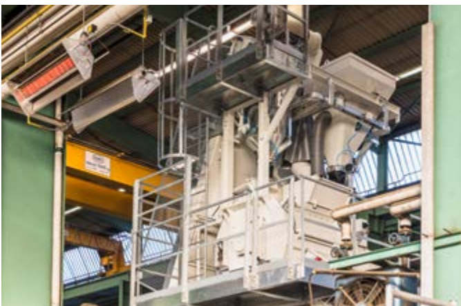
Good access to all plant components
