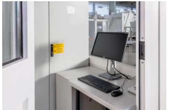
Integrated container with plant control system
